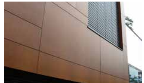
Fire station Saltaus, Italy Monolithic design, surrounded by nature. Projected by architects Menz + Gritsch.
